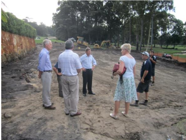
Figure 3 New putting green under construction (L-R Len Thomson, Michael Horne, Rod Davies, Lyn Smith)
